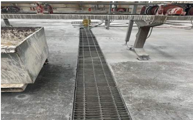
Plate 7 Factory centre with drainage to aeration pond
