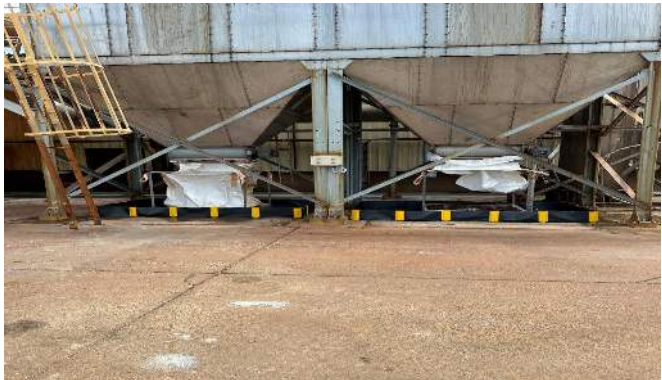
Plate 15 Lime bag house catchment
