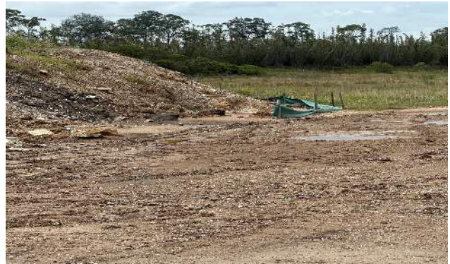
Plate 6 Stockpiles sediment fence requiring maintenance
