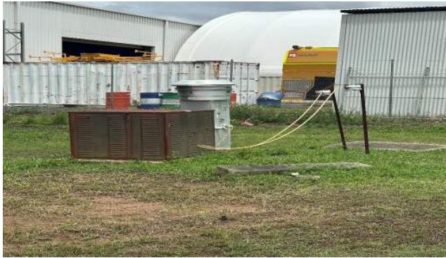
Plate 21 North Monitoring station
