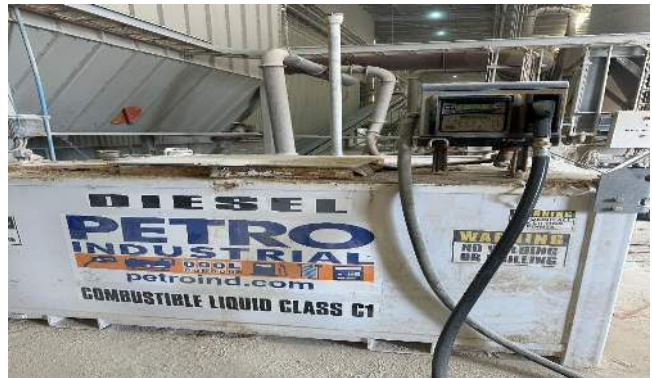
Plate 10 Diesel storage and refuel internal bund
