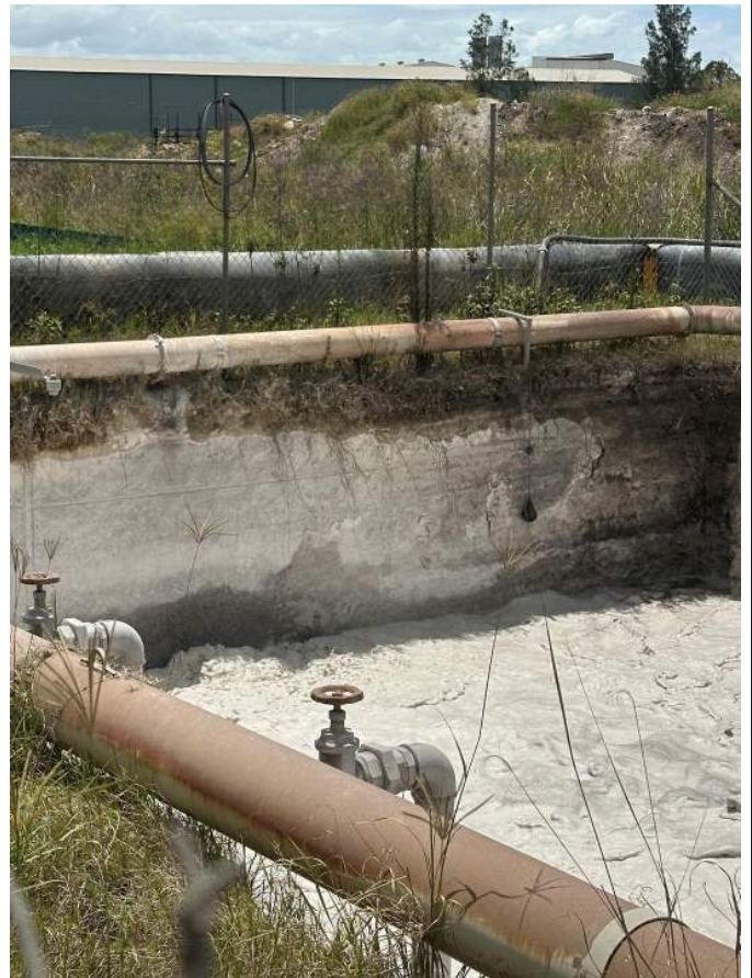
Plate 2 Aeration Pond Floating alarm and digital measure
